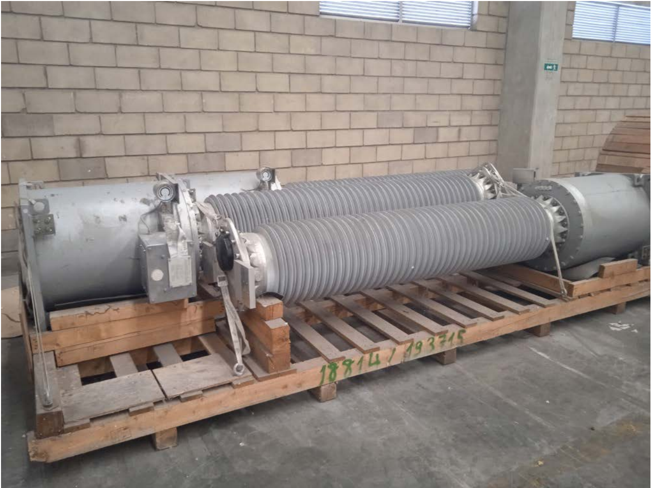
Figure 12: Substation parts storage status 1
