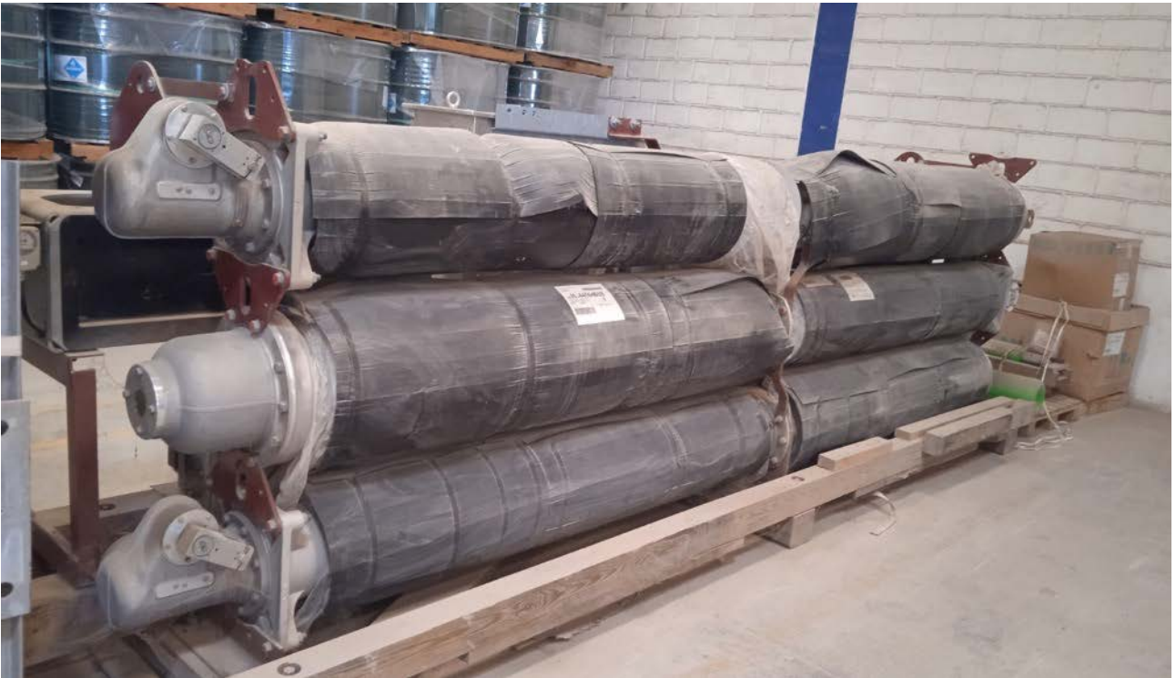
Figure 14: Substation parts storage status 3
